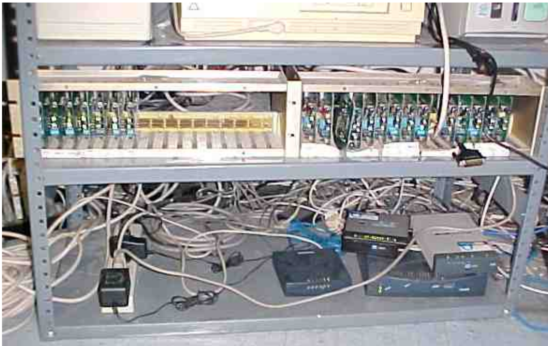
Figure 15. Typical rack of short haul modems, power supplies, and cables for DNC network driving 20 machines
